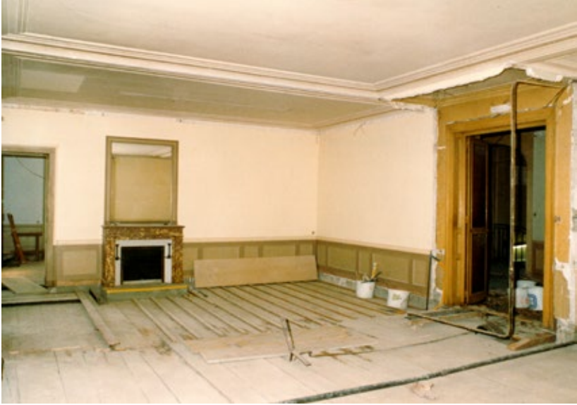
Renovation of rooms on the first floor Photograph, around 1986 Musée d'histoire des sciences
